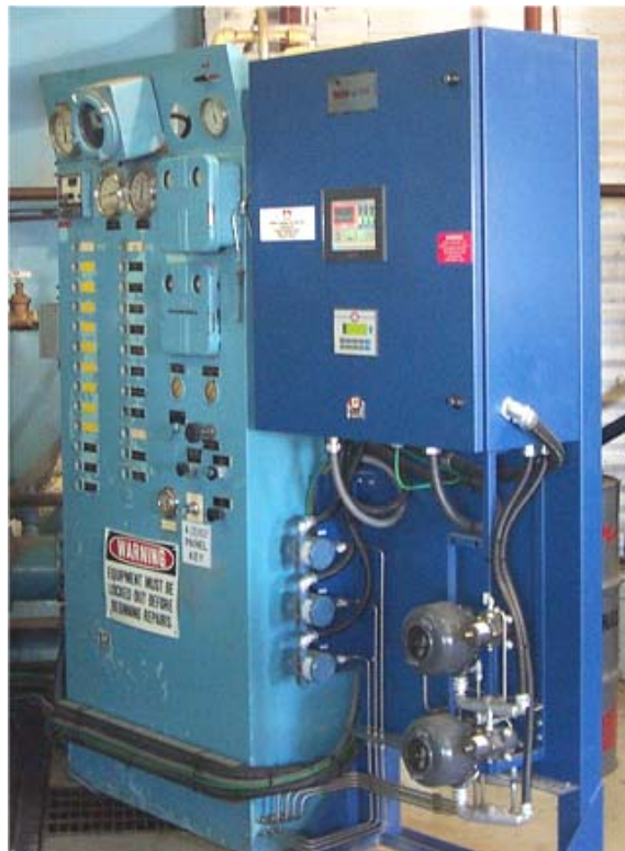
Old engine controller (left), and new REMVue® controller (right)
